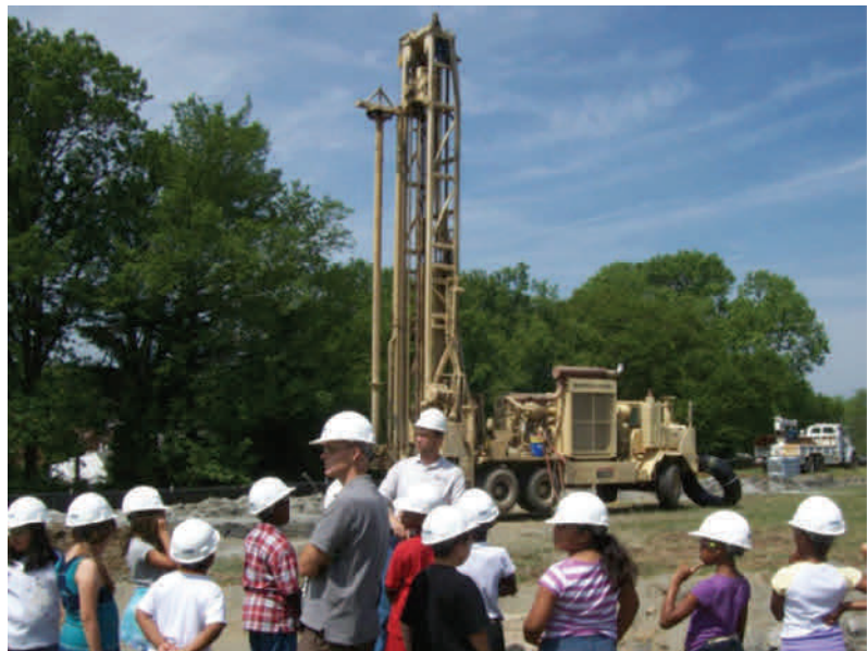
ACPS students observe the installation of the geothermal wells at James Polk ES as part of the school's philosophy of using green building initiatives as an opportunity for student education.
