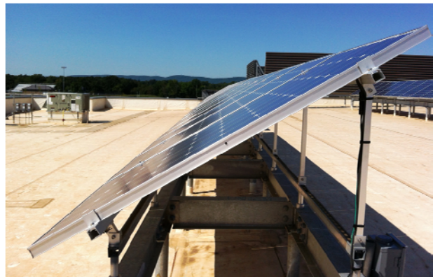
VIEW OF SOLAR PANELS
