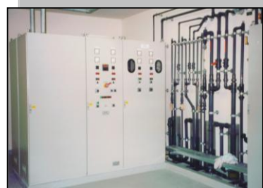
Corona discharge type ozone generator used in the five step pool water treatment process oxidizes germs and impurities in the pool. This saves chemical costs, reduces combined chlorine concentrations and provides more pleasant and less corrosive air and water conditions in the Natorium.
