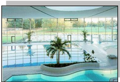
Leisure pool with ozone disinfection as part of the water treatment process. Palm trees live in the indoor environment and there is no chlorine odor.
